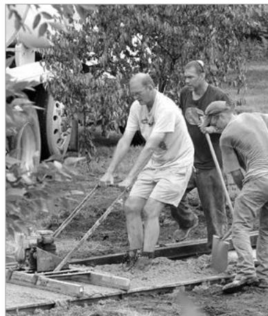
Staff members Gib Killion, Tim Jewell, and Clay Mankin pour a sidewalk to the new girls' dorm.
